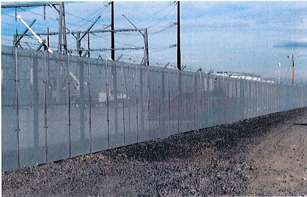
Example of Finished Fence: Expanded Metal panel with 5-strands of barbed wire
